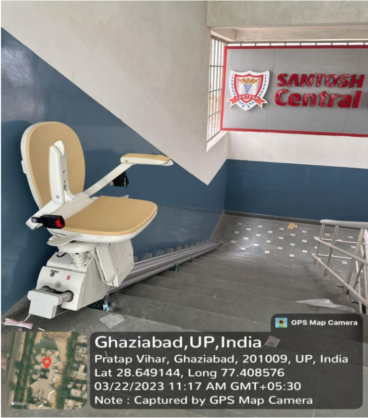
Stairs Lift for person with Disabilities
