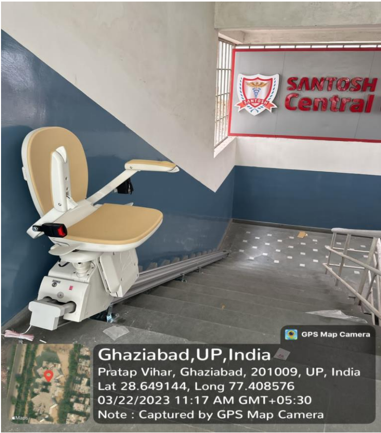
Stairs Lift for person with Disabilities
