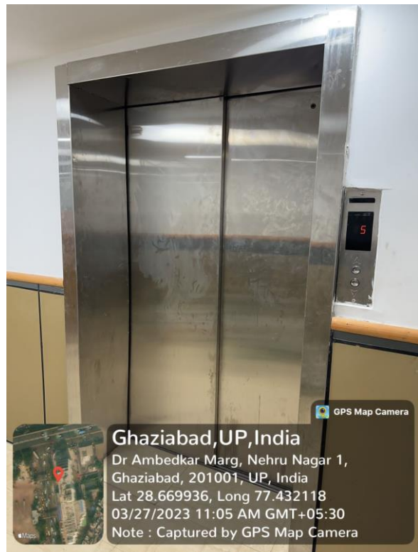
Patient Lift Hospital Building
